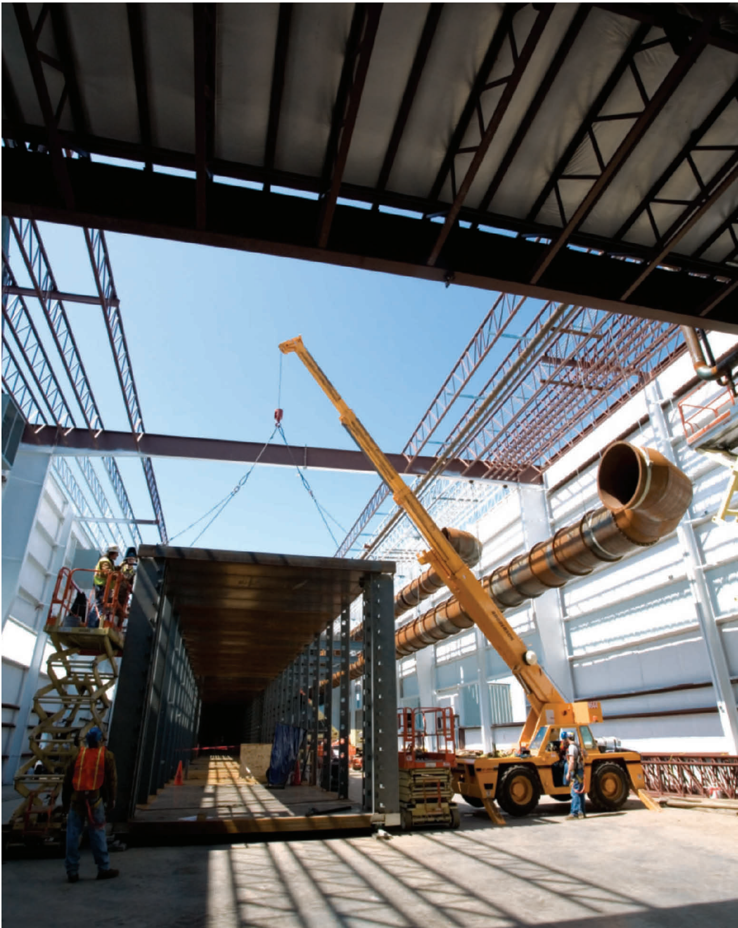
Installation of the dryers. The dryers that are installed at our Georgetown, South Carolina, wallboard plant are efficient and of significant size.
