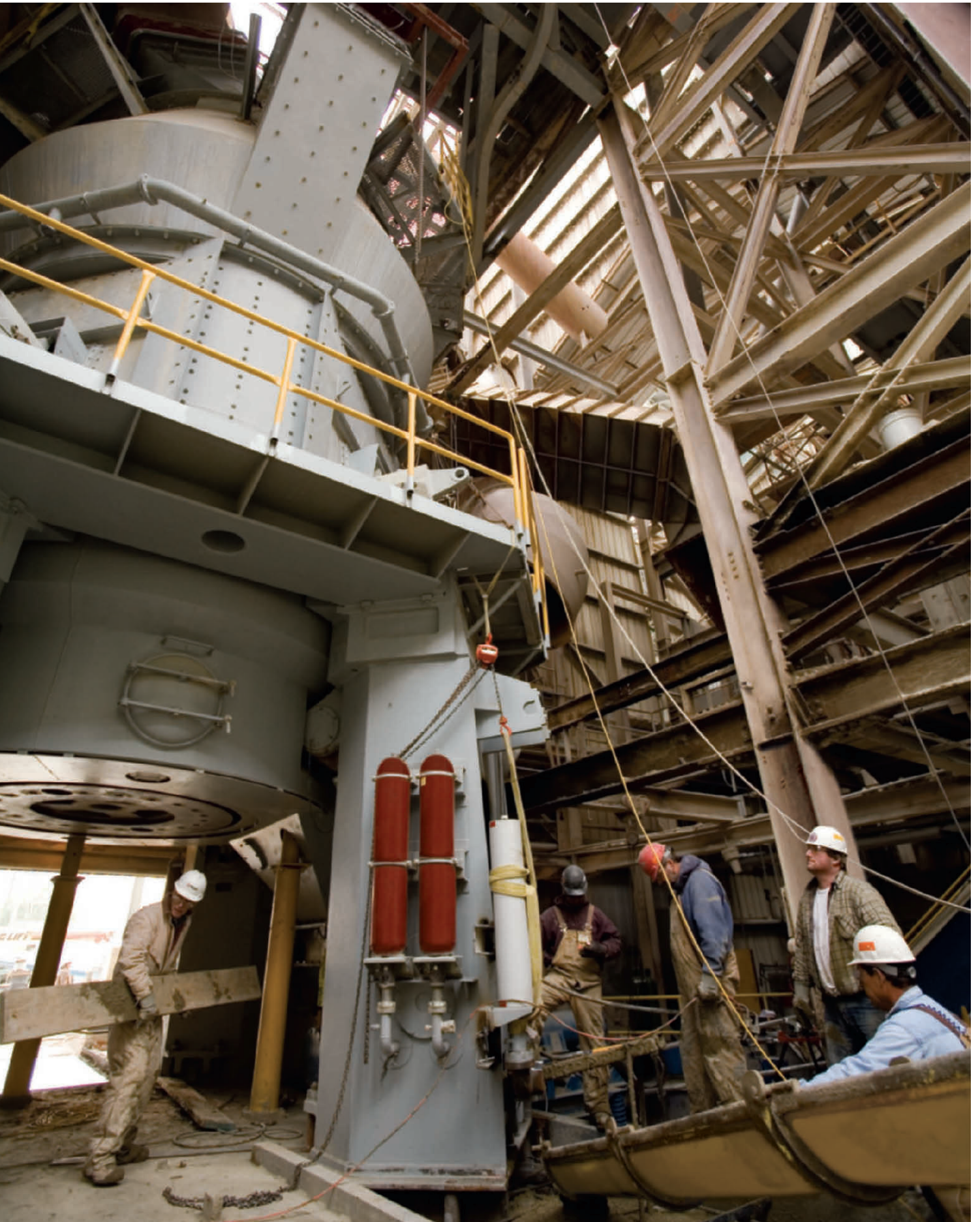
We used an innovative "slide-in" approach to install this massive new raw mill at our Illinois Cement facility. The new raw mill will play a vital role in reducing the operating costs and improving the throughput of the entire cement manufacturing process at Illinois Cement.
